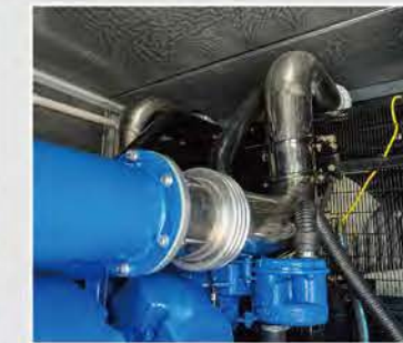
Interior of the genset
